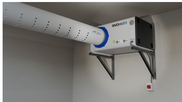
Wall mounted with airhose inside growing area
