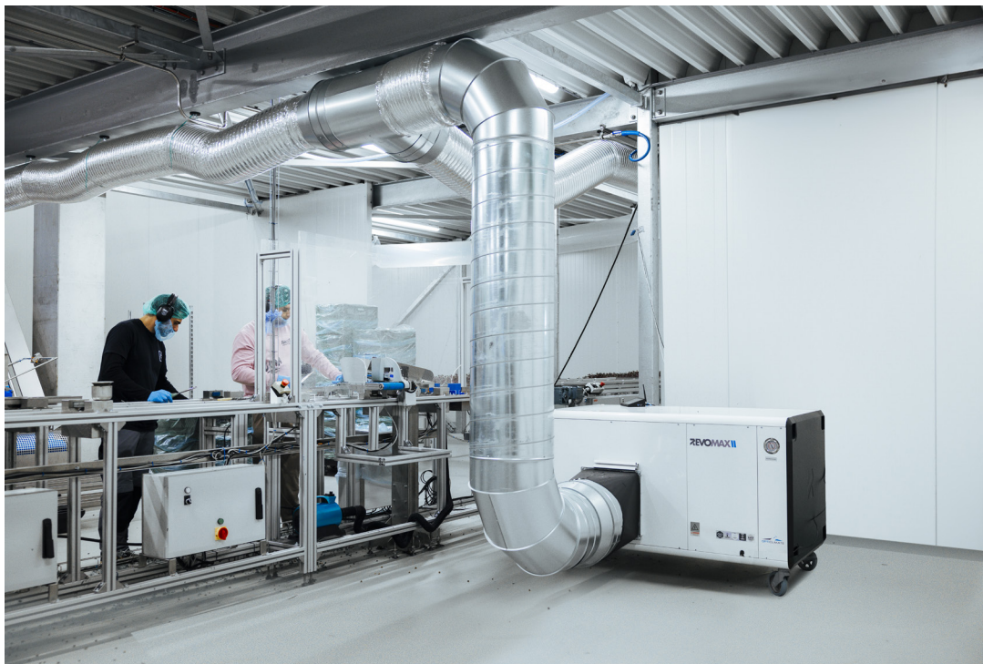
RevomaxII sep-fan and custom aluminium airhoses. The fan is installed integrated in the airhoses.
